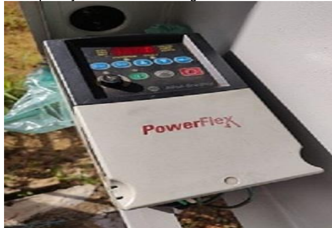
Figure 4 - Frequency inverter used to regulate the rotation of the fan rotor
