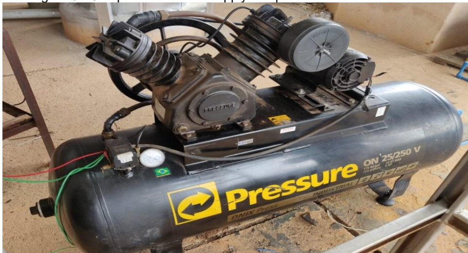
Figure 6 - Compressor used to supply compressed air to the vortex tube
