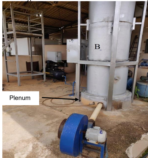
Figure 1 - Prototype silo used to evaluate the artificial cooling system
