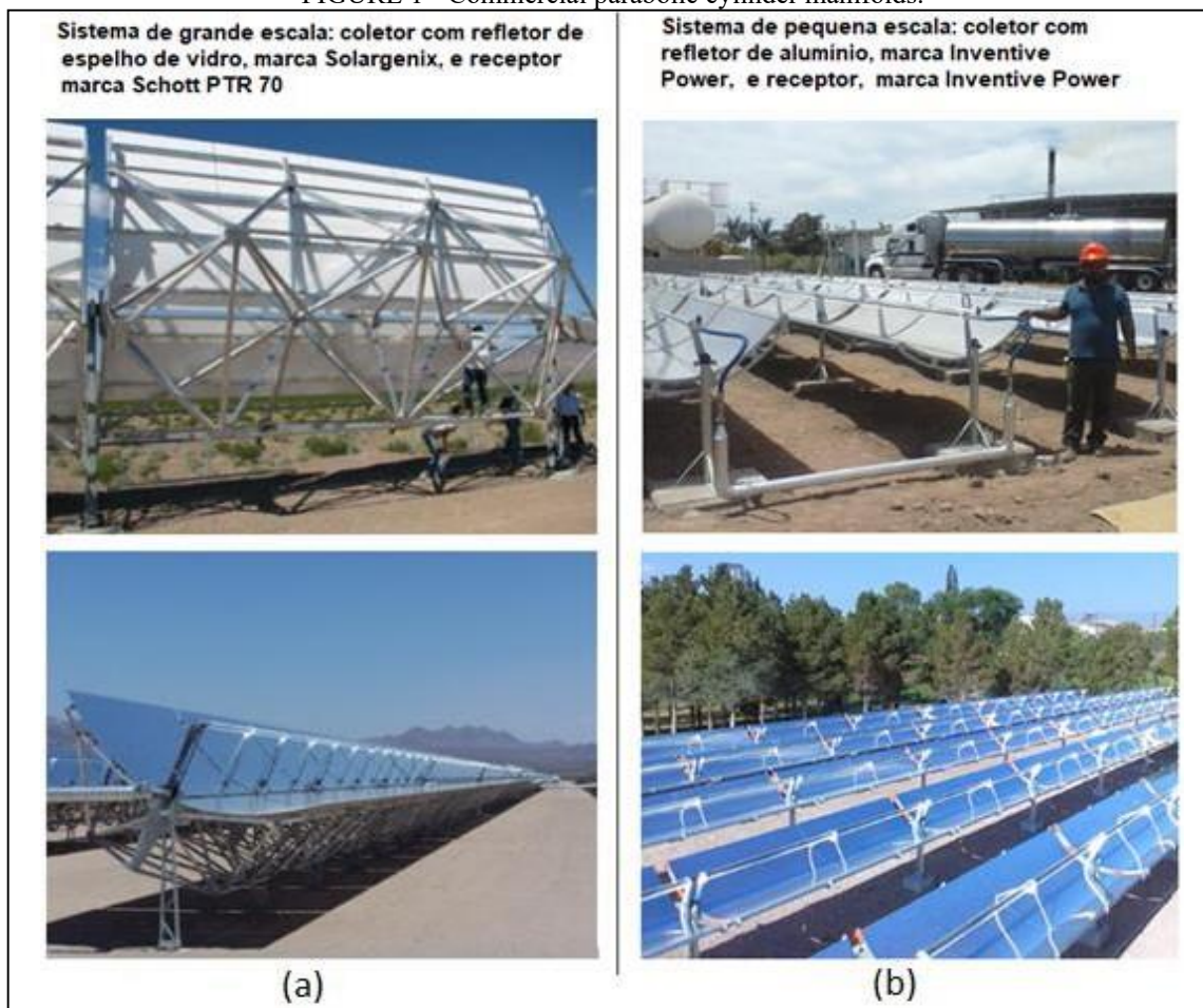
(a) Large collectors with Solargenix glass mirror reflective surface and Schott PTR-70 receiver. (b) anodized aluminum surface collectors and receiver, Inventive Power brand.
