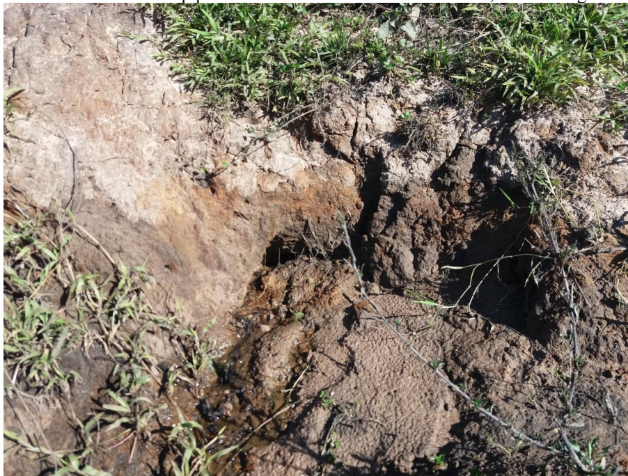
Figure 8 - Presence of an active pipeline with water flow on the riverbank, in the straightened section.
